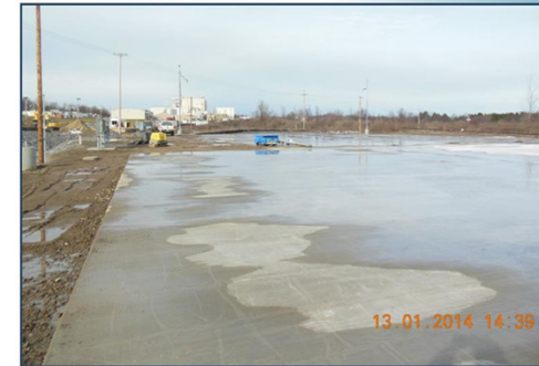
Five separate concrete placements and more than 300 concrete deliveries were involved in completing the HLW Storage Pad and Approach Apron.
