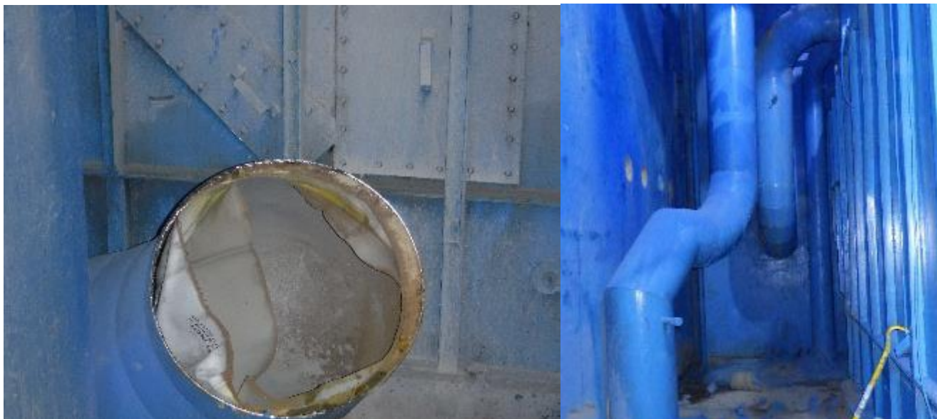
(Left) View of the vent duct after being cut with a diamond wire saw and (Right) duct sections to be cut
