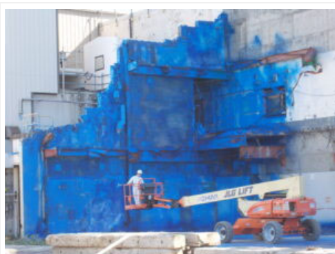
A worker at the West Valley Demonstration Project applies Polymeric Barrier System (PBS) to the concrete wall of the former main plant office building to protect employees from potential hazardous materials and unintended releases.
