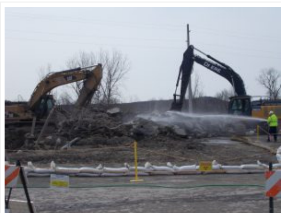
Two large excavators create work efficiencies as one demolishes the structure and the other size-reduces and loads debris.
