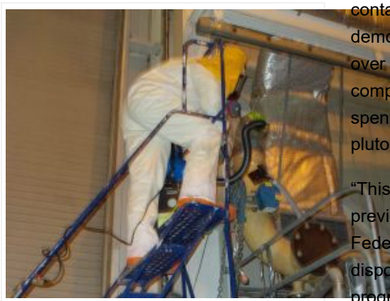
An operator, inside the fuel receiving and storage facility at the West Valley Demonstration Project, pumps a fogging agent inside a pipe to fix suspected contamination. This work was part of the deactivation of the FRS, along with the removal of asbestos-containing material.
