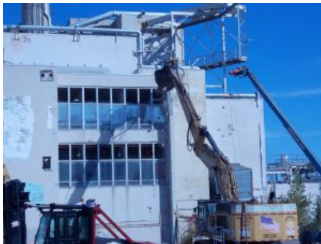
A large excavator, with a shear attachment, takes the first bite out of the main plant office building at the West Valley Demonstration Project.
